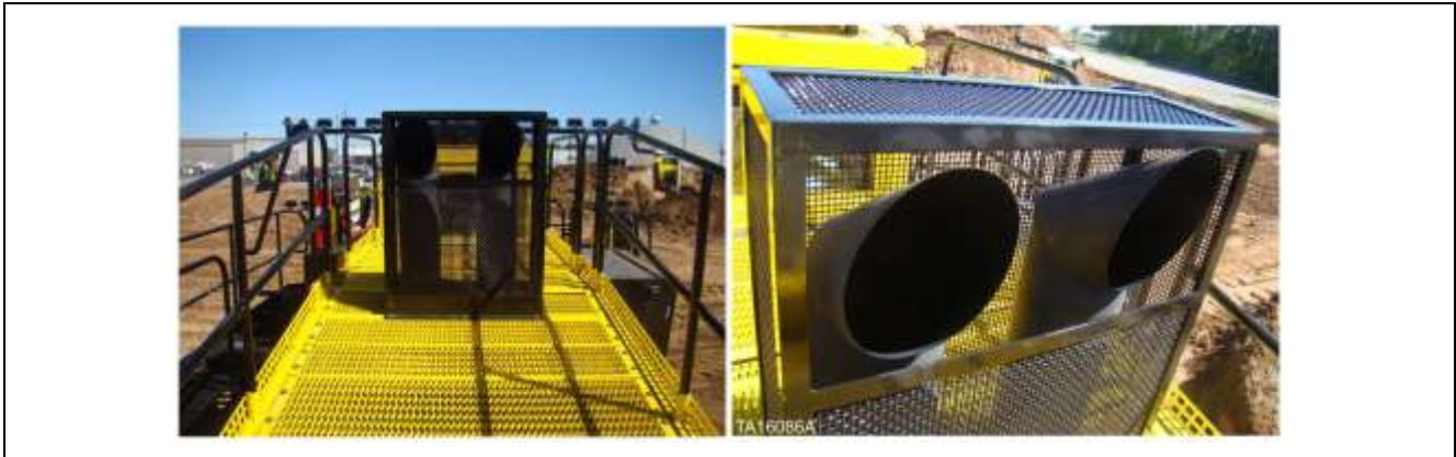
Figure 19. Engine exhaust stacks guard assembly
